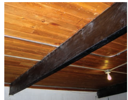
A retrofitted beam in the Coolidge Roundhouse gym is encased in a carbon-fiber covering.
